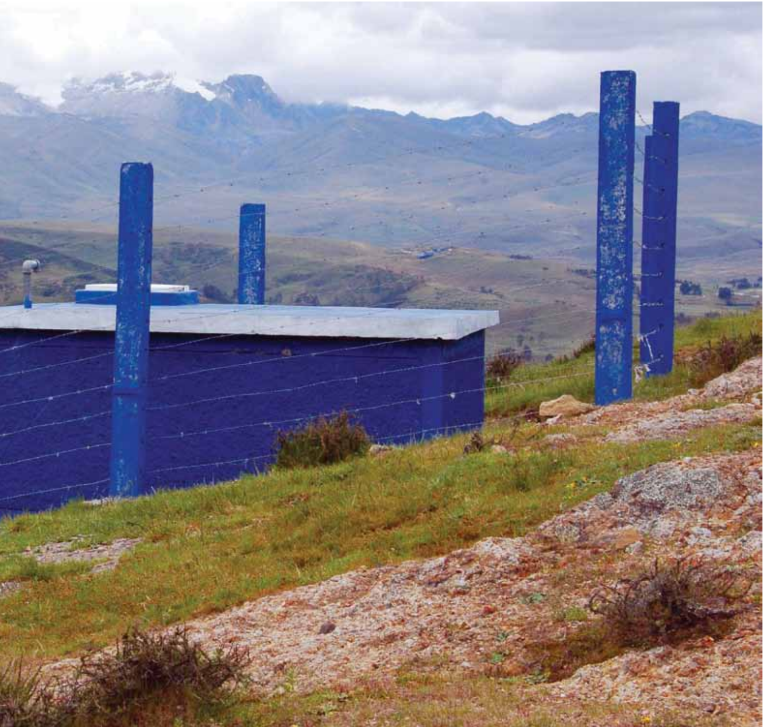
Yanamito water retention structure to store water during wet seasons for use in dry seasons.
